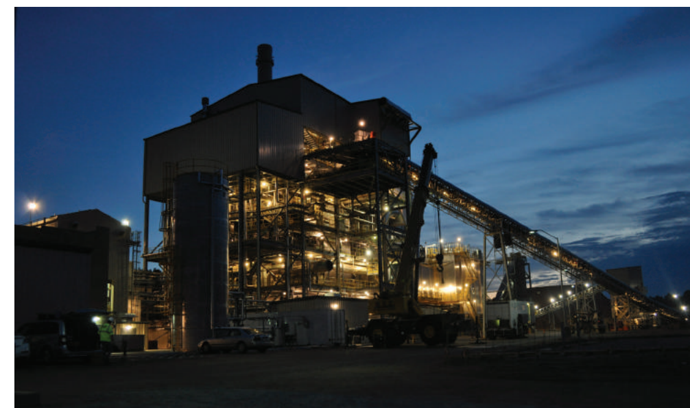
NOVEC's biomass electric generating facility in South Boston, Va.
